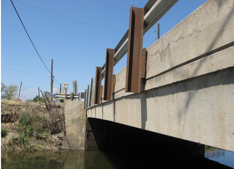
Photo 21. Existing E. 88th Avenue Bridge abutments within the prism of the O'Brian Canal, view to east.
