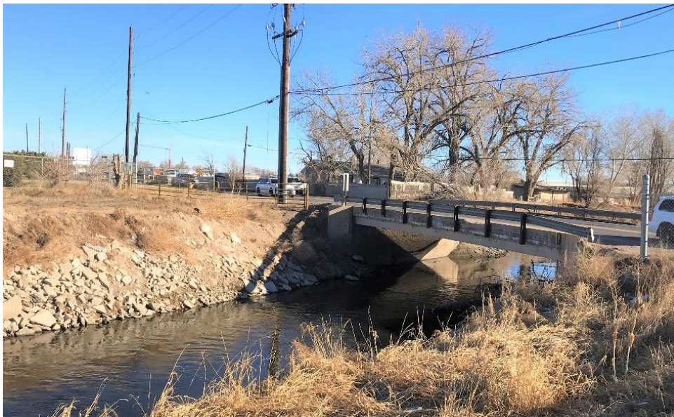
Photo 20. 5AM.477—O'Brian Canal. View south toward E. 88th Avenue Bridge. This recent photo shows the bridge abutment within the canal prism and the riprap added to canal banks in 2019, view to east-southeast.
