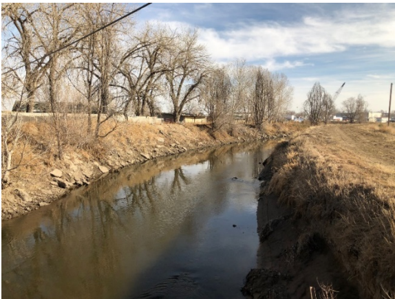
Photo 2. O'Brian Canal (S-1) crossing under E. 88th Avenue within the project study area (looking south).
